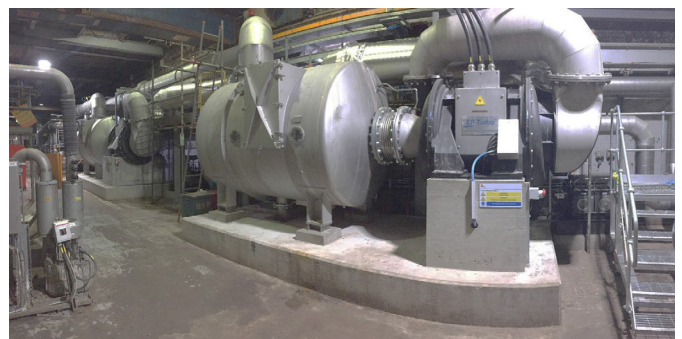
New EP600 Turbo blowers installed behind the machine.
